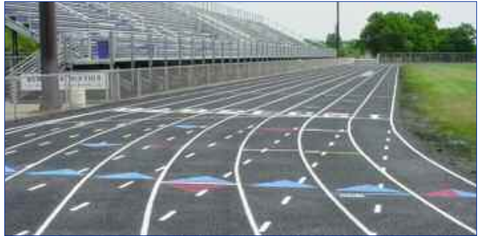
Asphalt surfaces are common on school grounds for drives, parking lot, and trails. Here the base course for a high school running track is being laid. The finished surface will eventually be a crumb rubber bonded together with either a latex or polyurethane binder. The finished marking are applied following very exacting dimensions and specifications.
