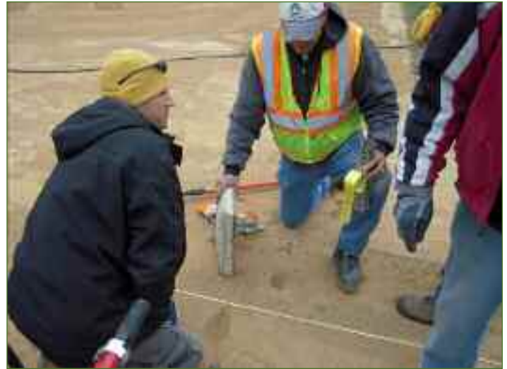
Josh Graham, left, a sports turf manager at TCF Bank Stadium at the University of Minnesota, and Chad Maata, City of Prior Lake, volunteered their time to help renovate a baseball field in Farmington, Minn.
