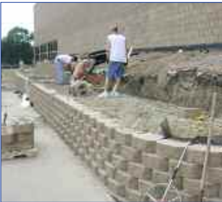
The life of a school requires upgrades and replacements to landscape features that have failed or have served their useful life. Above, a timber retaining wall is being replaced with a concrete segmental retaining wall system.
